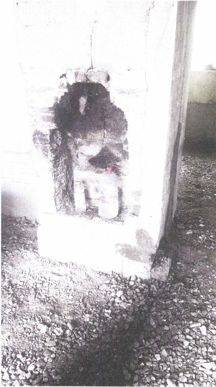
Chimney with multiple cracks crack all the way up center, no lintel, crack also to right.
